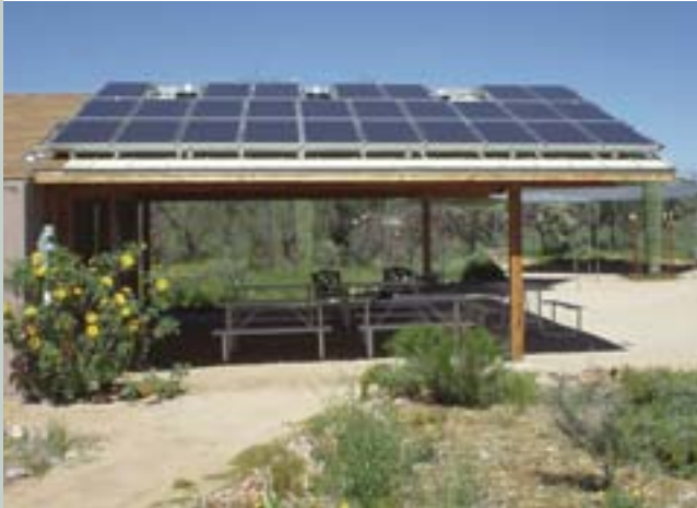
The Audubon Society's Mason Center uses solar energy thanks to Tucson Electric Power and its customers.
